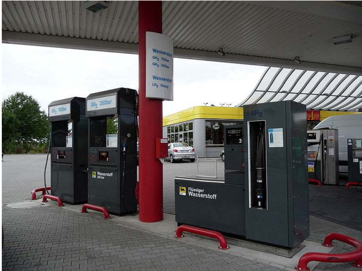
Hydrogen filling station near Frankfurt, Germany. Picture in public domain.
